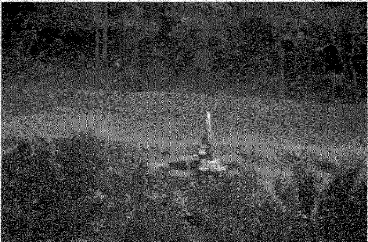
Figure 4. This photo was taken by Dean Wilson during a monitoring flight on July 23, 2018. This photo depicts the pipeline right of way as it crosses the Property. As seen in the photo, there is construction equipment, one excavator, on the Property indicating active construction thereon.
