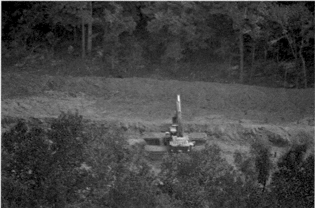
Figure 4. This photo was taken by Dean Wilson during a monitoring flight on July 23, 2018. This photo depicts the pipeline right of way as it crosses the Property. As seen in the photo, there is construction equipment, one excavator, on the Property indicating active construction thereon.
