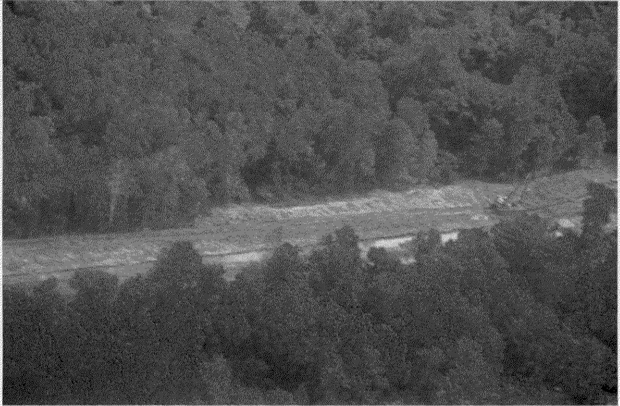
Figure 3. This photo was taken by Dean Wilson during a monitoring flight on July 23, 2018. This photo depicts the pipeline right of way as it crosses the Property. As seen in the photo, there is equipment on the Property and it appears that the trench in which the pipe will be laid is being dug along the pipeline route as it crosses the Property.
